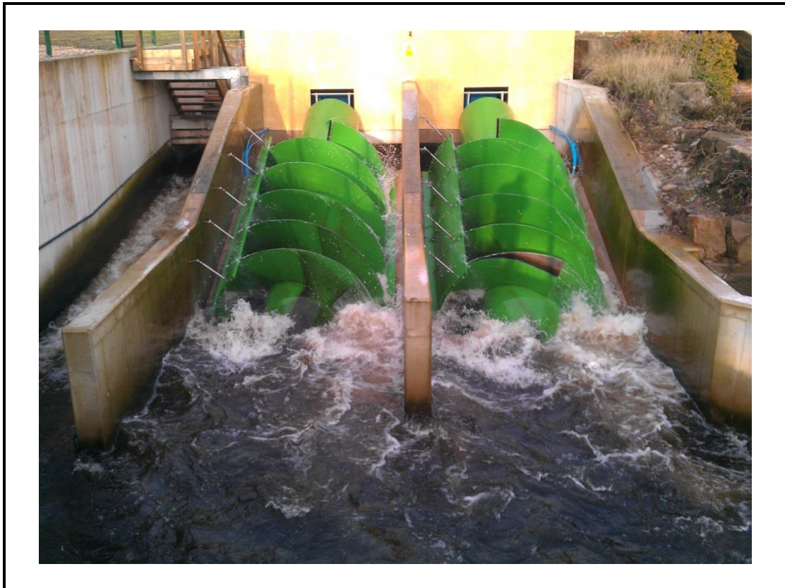
Figure 3.2: Photograph of the twin Archimedes Screw Turbines at Otterspool weir
