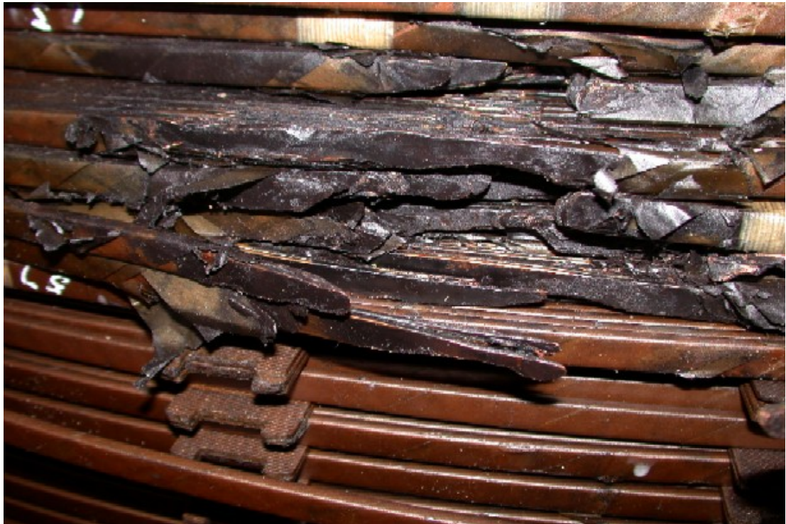
Figure 2: Failure in a large South African generator transformer three weeks after the Halloween storm of October 2003. The disruption of the winding and insulation by the arcing fault at the time of final failure is clear. The arcing fault also destroys evidence that might lead to a better understanding of the progression of damage after initiation by the geomagnetic current event.
