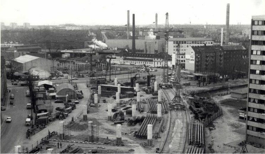
Figure 6.20: Bispeengbuen under construction showing how it cut a swathe through the existing neighbourhood SOURCE: City Archive 50675
