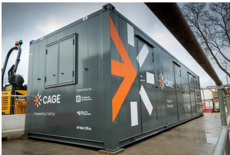
Figure 5.1.2 - Photograph of LPG engine in welfare cabin at HS2
