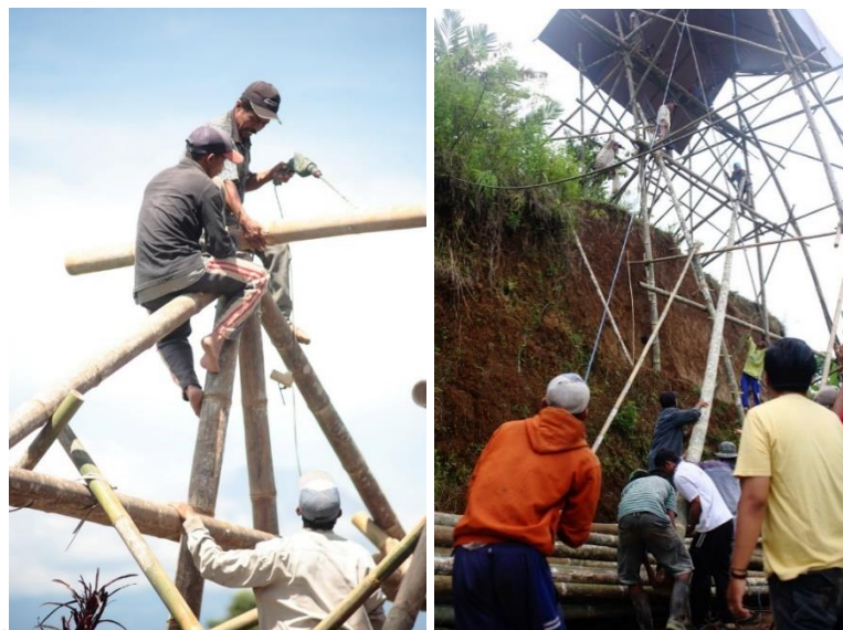
Figure 15: Prototyping phase. People erected the bamboo tower on the future site of the church (ASF-AD, 2016)
