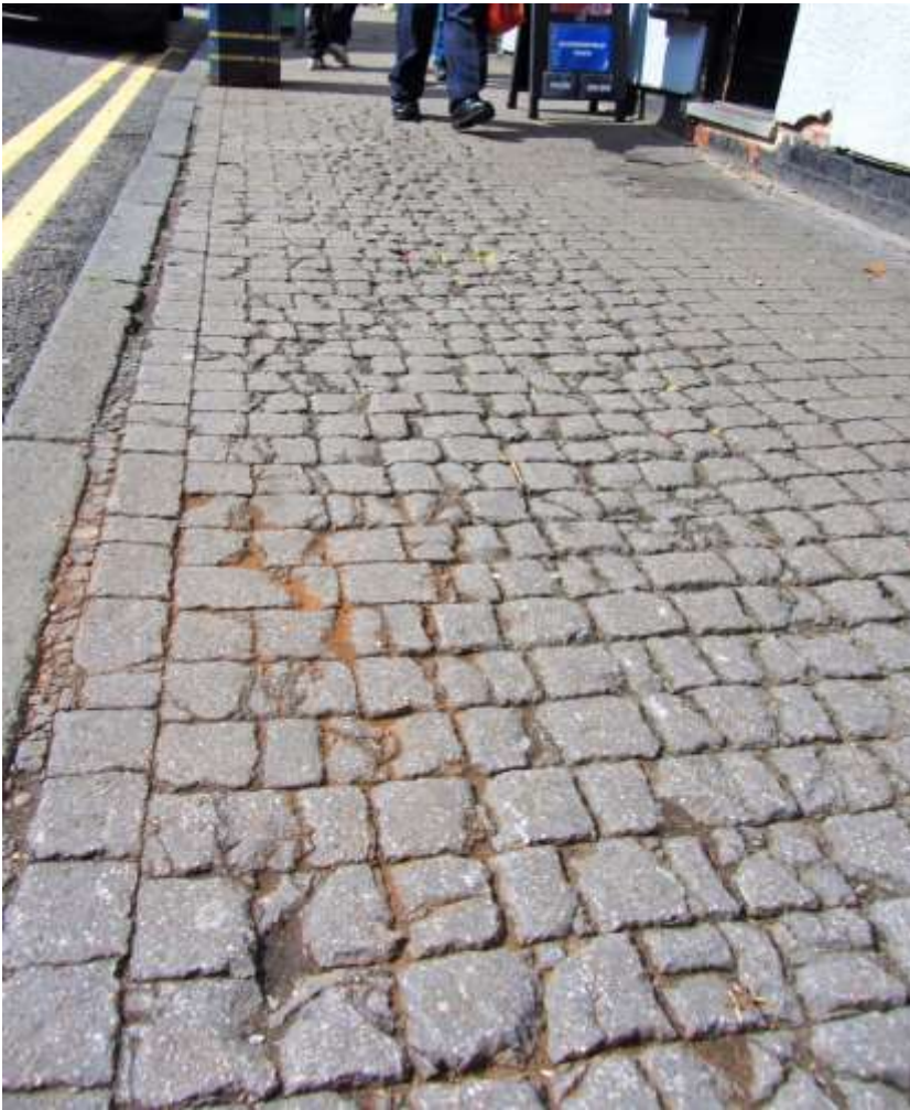
Figure 3. An uneven and broken section of the pavement on Harborne High Street that caused participants discomfort and led to undue exertion and exhaustion (JB).
