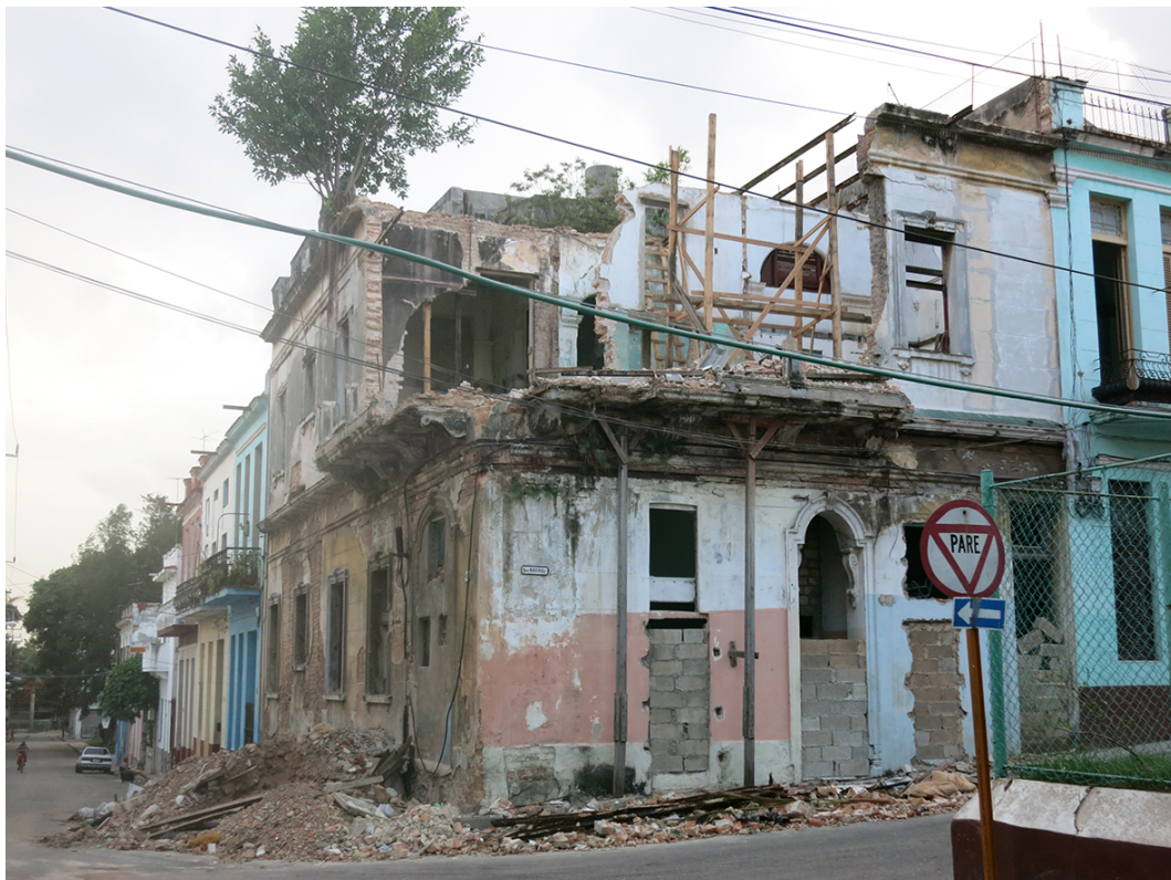
The common sight of a recent partial building collapse, marked by the rubble piled in the street, El Vedado, Havana, 2017.
