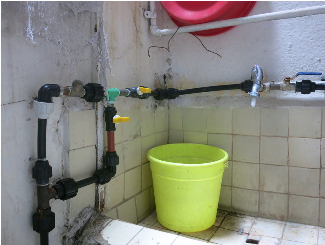
The complex plumbing configuration works by opening and closing stop taps at strategic points of each day, Central Havana, 2016.
