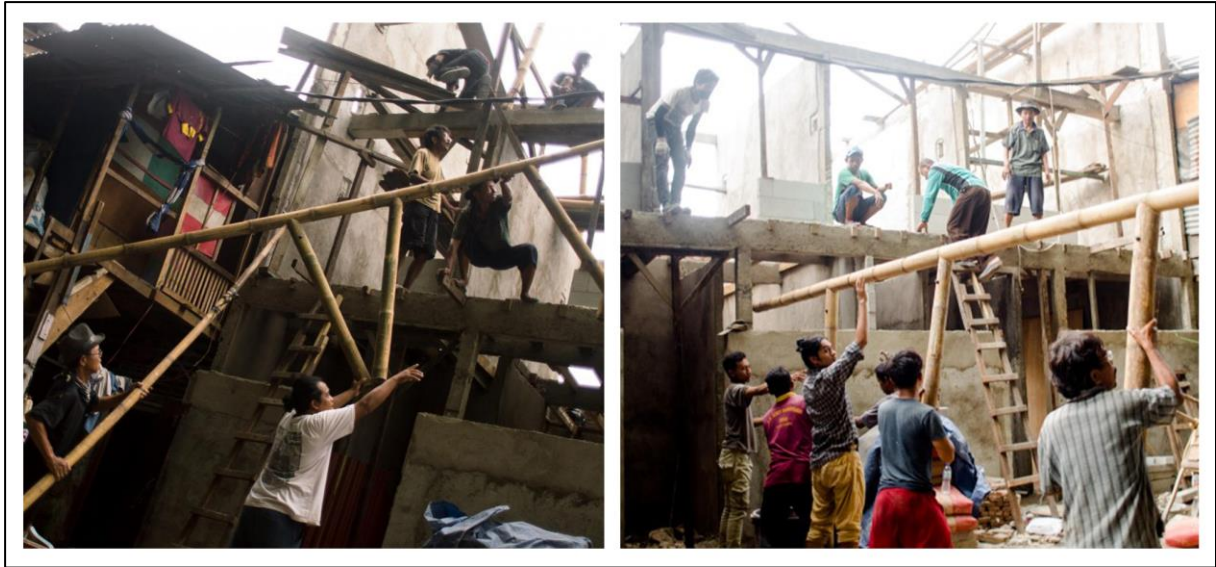
Figure 1 The building process of the prototype house project in Jakarta conducted by involving the residents and designers. Image reproduced with permission of the rights holder, ASF-ID (ASF-ID, 2015)
