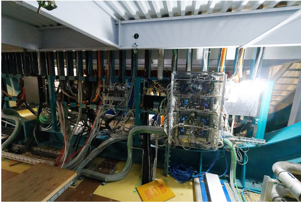
Figure 5.13: Cable trays to bring cables from outside the magnet to the basket. 16 of the 24 cable trays are used for the current tracker system and therefore only 8 cable trays will be available for the new subdetectors.
