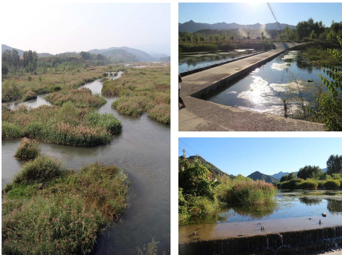
Figure 6.9 Photo of eco-purification of Chao River in Beijing, China. Bulrush and reeds extract phosphorus from the river. Weirs retain the water in a sequence of basins while the ecosystem cleans the water of impurities. Water is aerated upon exit to increase the amount of oxygen dissolved in the water.
