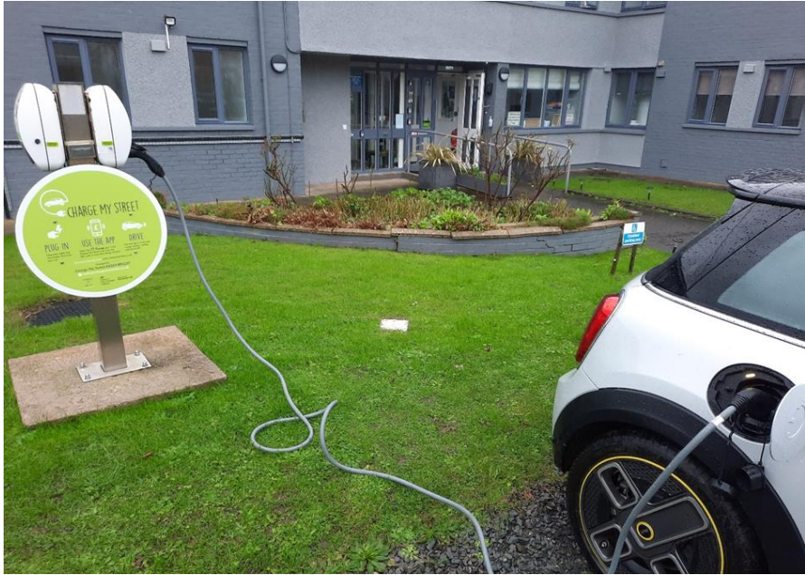
Figure 24 - West Point House chargepoint, as seen in map format at in Figure 22.1. Taken by E., Dolmor
