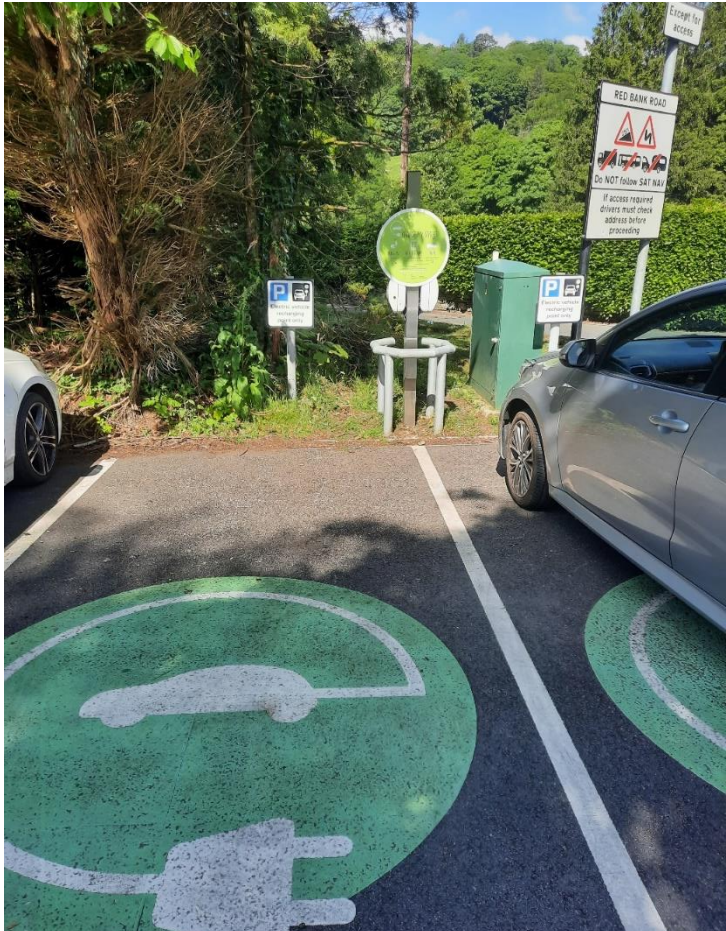
Figure 25 - Red Bank Road Car Park Chargepoint, as seen in map format in Figure 22.2. Taken by E., Dolmor
