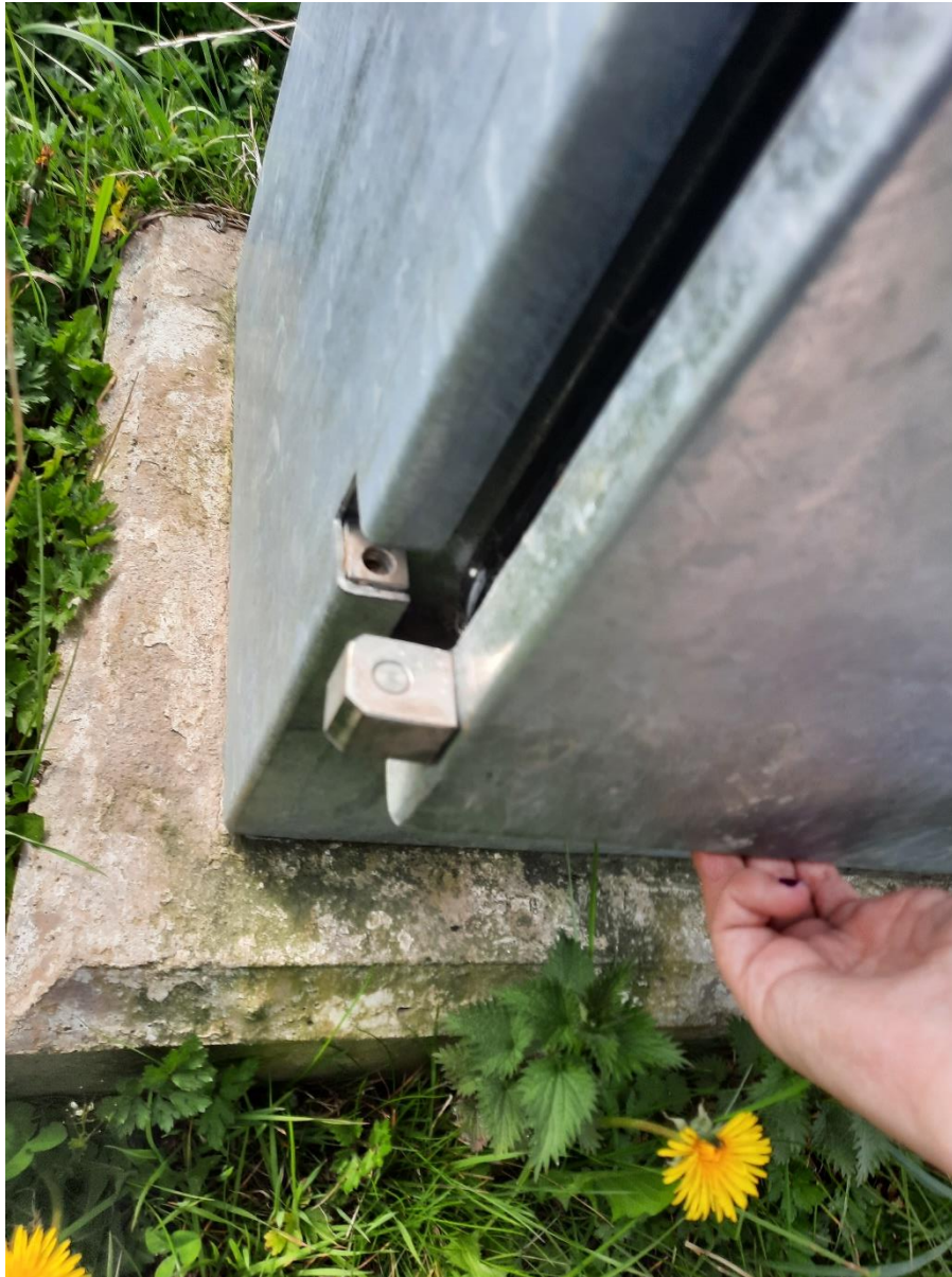
Figure 9 - Chargepoint Fuse Cupboard broken door in Cumbria. Taken by E., Dolmor.
