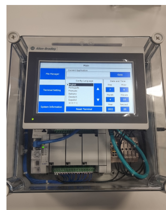
(c) Allen Bradley MicroLogix 850 and HMI in box
