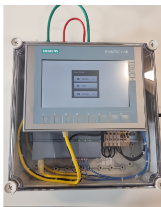
(b) Siemens S7-1200 PLC and HMI in box
