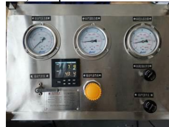
c) Pressure controller
