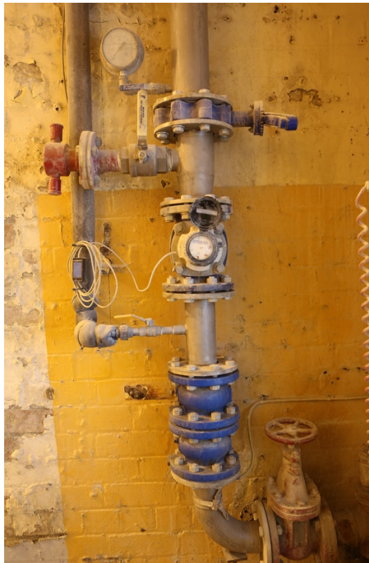
Figure 76: The water meter for Crown Paints' Darwen Emulsion Plant.
