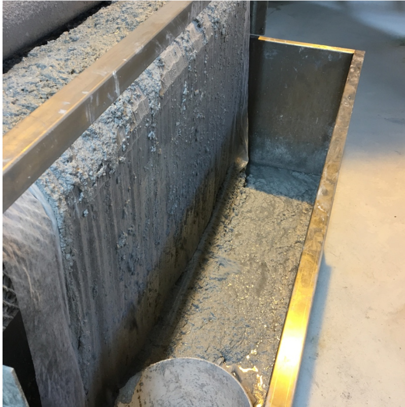
Figure 157: Quantity of sludge being removed via the Bandfilter.
