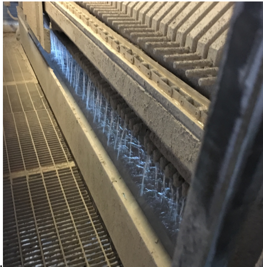
Figure 119: The Hull effluent plant filter press dewatering.
