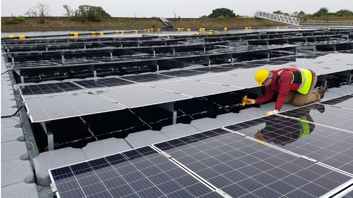
Figure B-2 – Water depth being recorded at an under array location. Each under array location had a metal chain attached to the underside of the FPV array, supporting HOBO Pendant® temperature loggers at 0.5, 1, 3 and 5 m.
