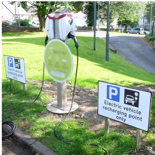
Figure 46: Charge My Street Installation
