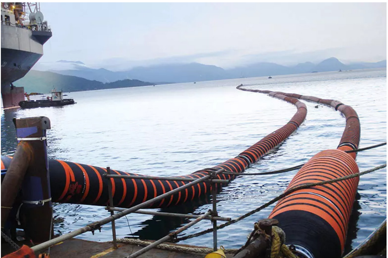
Figure 1. Trelleborg’s Sealine floating hose during installation to a supply vessel. (Sealine is a product type that is specifically designed for floating hose configurations, while Reeline is a product type that is specifically designed for reeling hose configurations. Both Sealine and Reeline are hose products made by Trelleborg, a hose manufacturer. Courtesy: Trelleborg; adapted with permission.).
