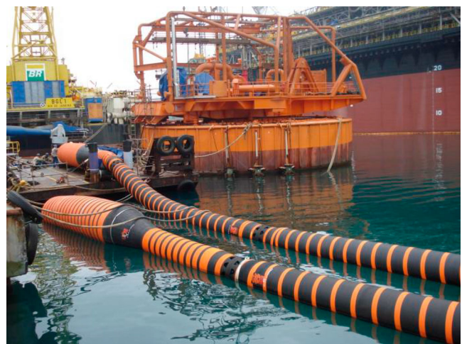
Figure 19. Installation of floating hoses for a CALM buoy in offshore Brazil (Courtesy: BR) (This figure is available in colour online).
