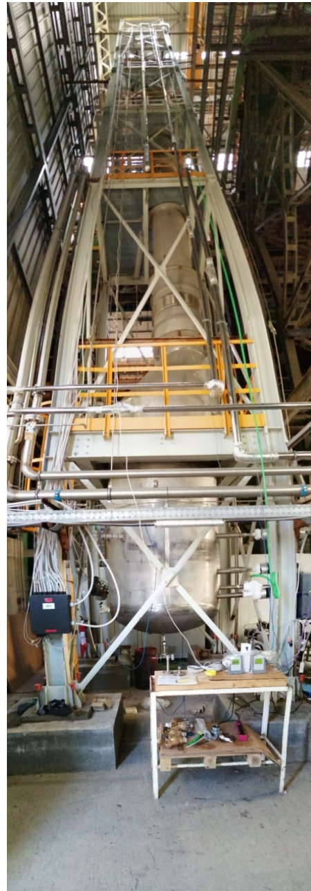
Fig. 10 The prototype Aria plant in the Laveria building of the Carbosulcis mine, Nuraxi-Figus site, viewed from the basis of the column.
