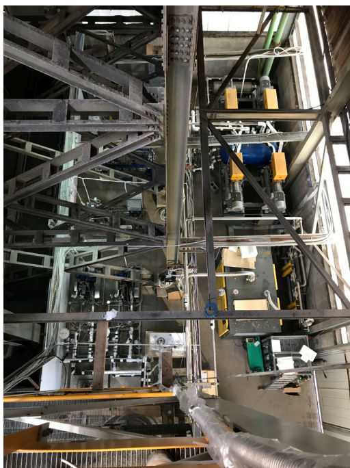
Fig. 11 Aerial view of the prototype Aria plant located in the Laveria building of the Carbosulcis mine, Nuraxi-Figus site. From bottom left, clockwise, the liquid pumps, the cryocoolers, and the gas compressor.
