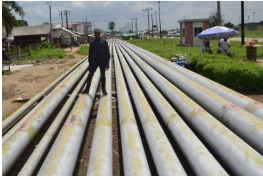
Figure 2.1. Pipeline showing violation of Right of Way (ROW) in Port Harcourt Suburbs, showing the author, taken during field survey in 2016.
