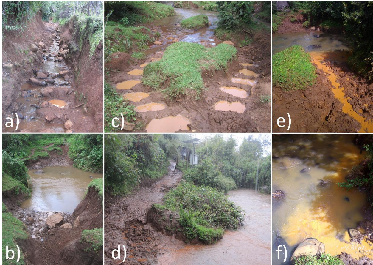
148 149 Figure 2 a-c) Incised and unpaved tracks provide a direct connection with the stream, d-e) degraded and 150 disturbed riverbank from livestock entering the streams and f) eroded suspended sediments in streams 151 within the smallholder agriculture catchment.
