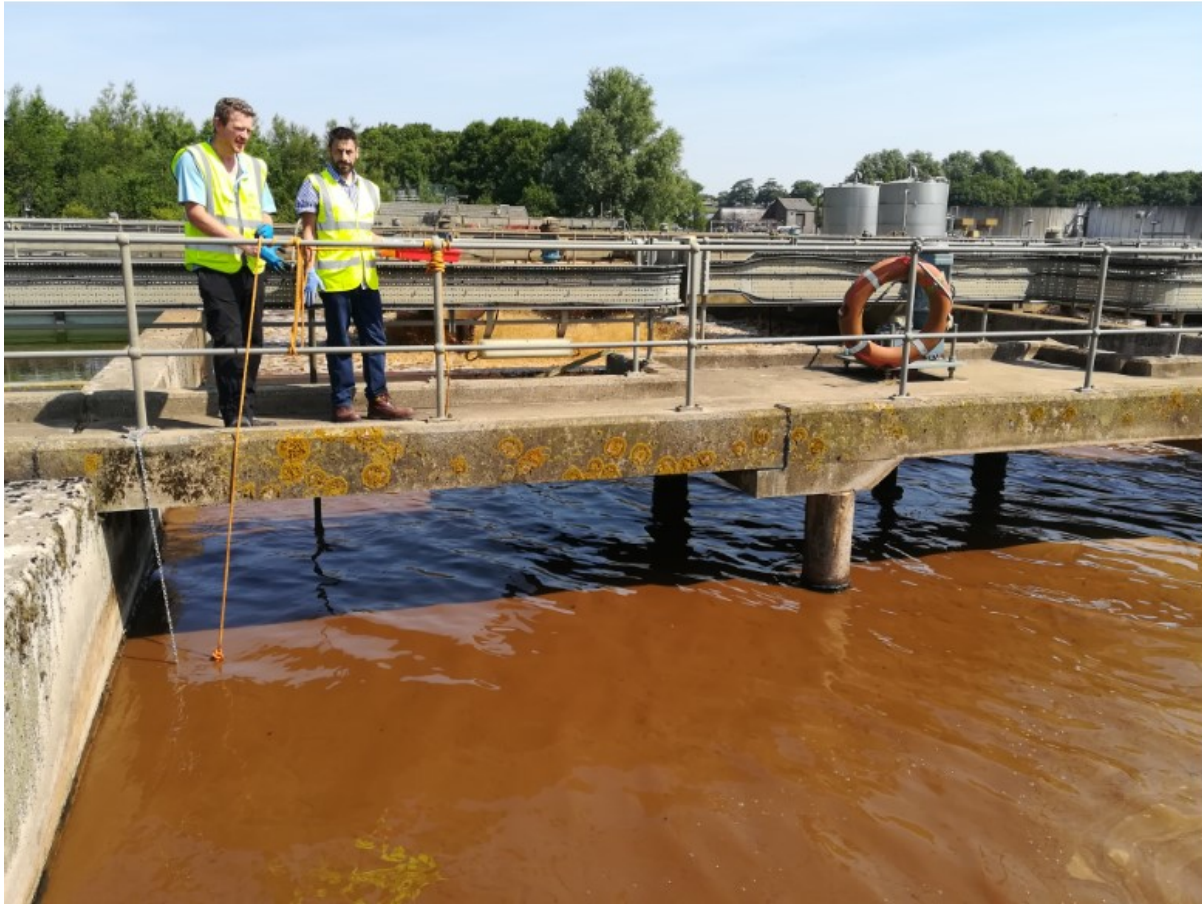
Figure 2: A section of Wastewater activated sludge plant.
