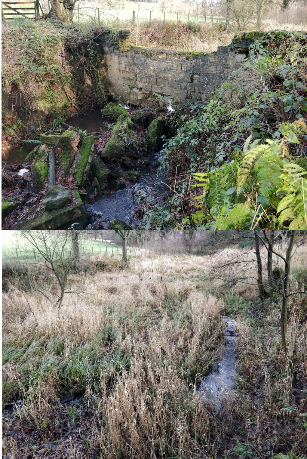
Figure 3.2.4. Photographs of the Redundant Pond potential hydropower site. Top: breached weir and stream leading to the Bull Ring. Bottom: Redundant Pond area and stream upstream of the breached weir.
