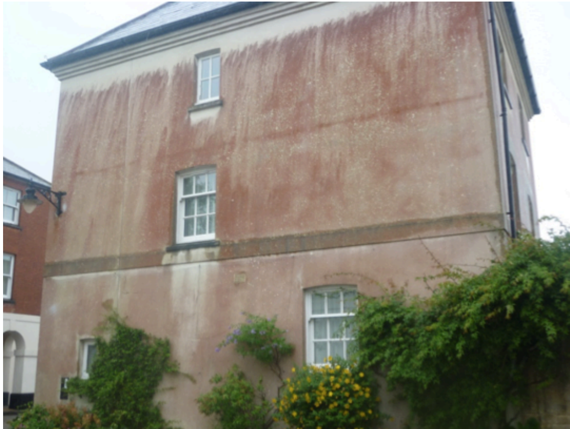
Figure 6.18: ‘Efflorescence on the exterior of Poundbury buildings’ which suggests cheap building materials. Photograph by author, July 2017
