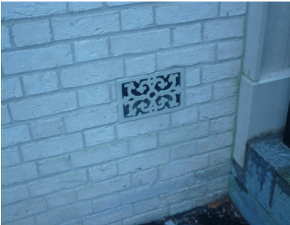
Figure 6.15: 'Concealed gas and installation pipes', on the exterior wall of a Poundbury building. Photograph by author, July 2017
