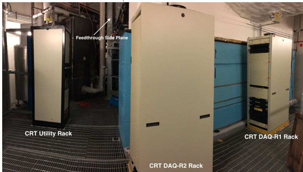
Figure 12: CRT racks in the LArTF pit. Three racks are located in a free area at the downstream beam end under the cryostat and next to the feedthrough side plane.
