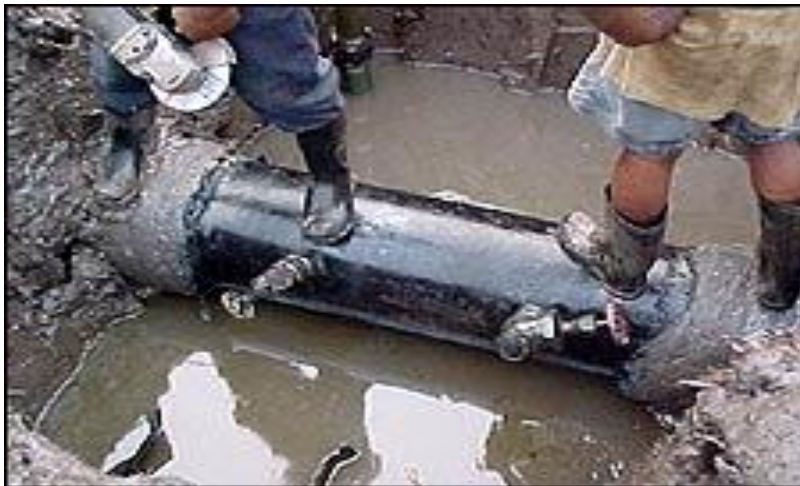
Figure 4.3: An illegal tap put in a pipeline
