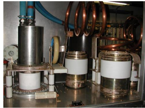
Figure 2.3. The main amplifier of one transmitter at EISCAT
