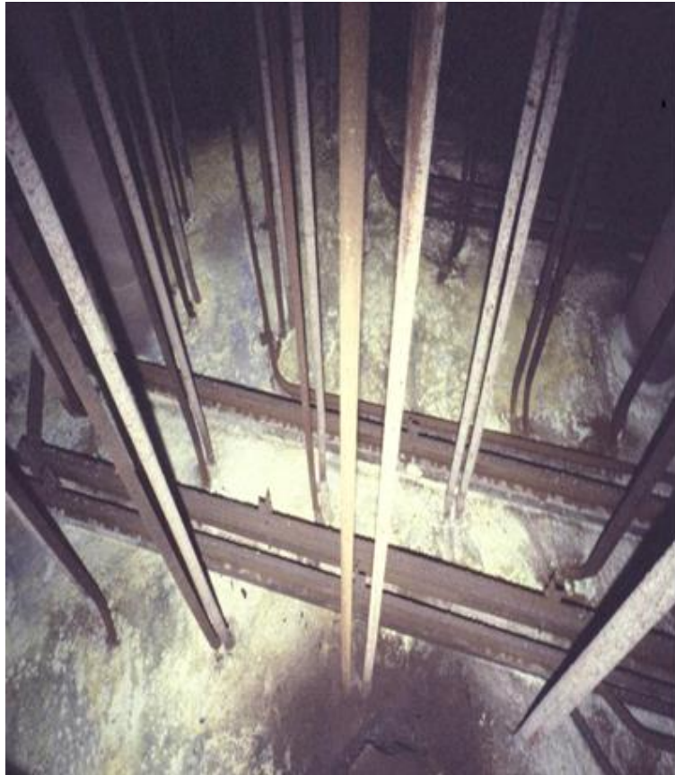
Figure 5. Example of the vertical and horizontal cooling coils in an SRS HLW tank.
